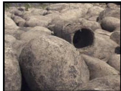
Close up of riverbed discharge diffuser head.
