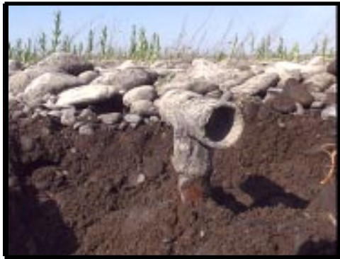
Riverbed discharge diffuser head located on the upstream tip of D-Island.
